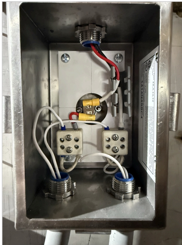
Figure 4. Interior of the secondary junction enclosure. Top: liquid-tight conduit fitting where the FMC bundle from the main enclosure enters; the red and black PTFE-insulated wires drop down to the snap disc. Center: snap disc thermostat (round disc, N.C., opens at 205°F, auto-reset) wired in series with the L1 heater hot path; yellow insulated crimp quick-connects secure the leads at the snap disc tabs. Lower left and right: ceramic high-temperature terminal blocks where TGGT-insulated heater leads (cloth-jacketed, white) transition to standard PTFE-insulated wires. Bottom: two liquid-tight conduit fittings where the heater leads exit toward the strip heaters. Hammond enclosure label (1414N4SSC4, Type 4X/4/13/12, IP66) visible at right.
