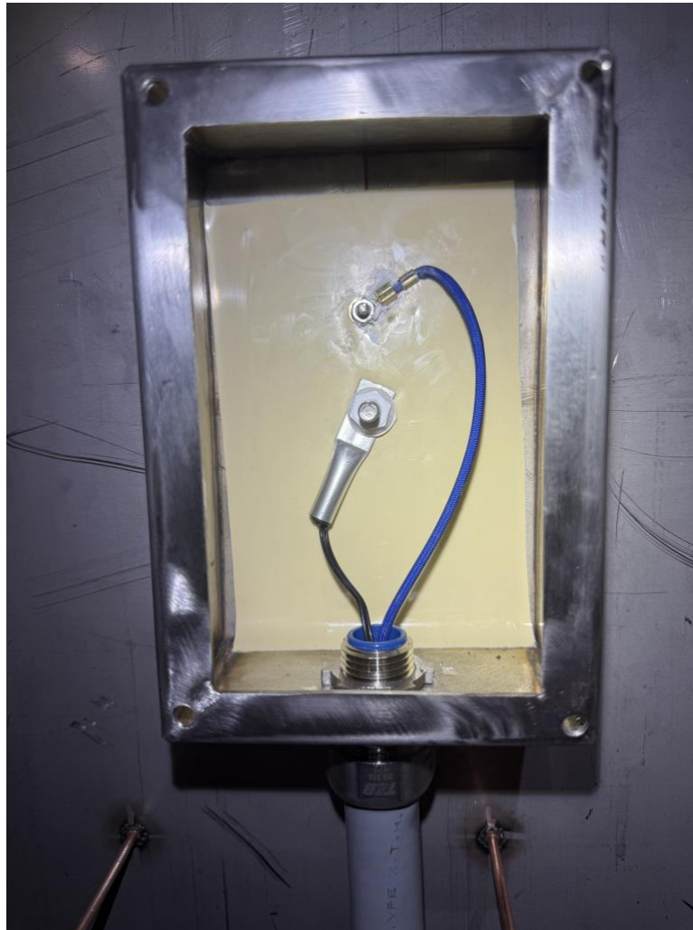
Figure 6. Redundant thermistor probe enclosure on the tank exterior. Two lug-style probes are bolted to the stainless tank wall through silicone thermal pads (visible cream-colored backing). The blue-jacketed loop is the nickel plated copper lead from one probe; the second probe attaches at the lower-left lug and is aluminum galvanically separated from the stainless steel tank. Probe leads exit through a liquid-tight conduit fitting (right) and return to the controller via the vapor-tight FMC. Disconnect both leads before measuring resistance using the table in Section 4.4.
