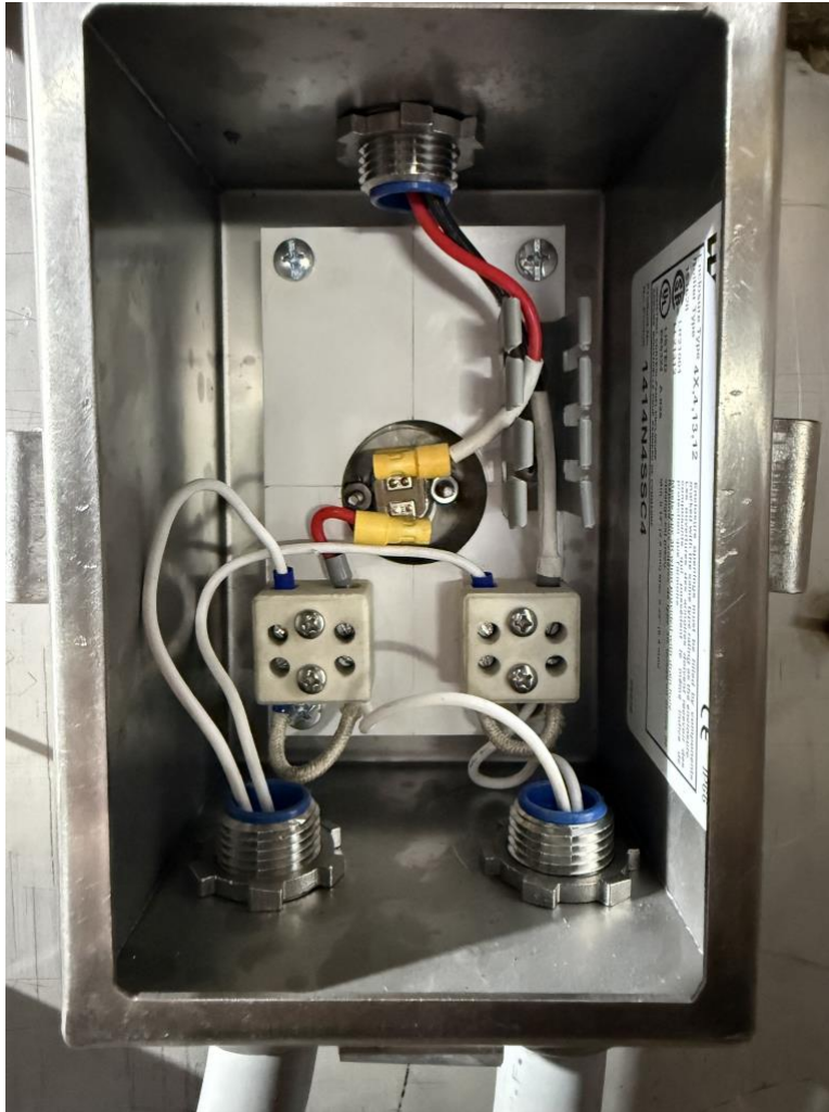
Figure 5. Interior of the secondary junction enclosure. Top: liquid-tight conduit fitting where the FMC bundle from the main enclosure enters; the red and black PTFE-insulated wires drop down to the snap disc. Center: snap disc thermostat (round disc, N.C. opens at 200^{\circ}\text{F} \pm 5^{\circ}\text{F} ) wired in series with the L1 heater hot path. Lower left and right: ceramic high-temperature terminal blocks where TGGT-insulated heater leads (cloth-jacketed, white) transition to standard PTFE-insulated wires routed back to the main enclosure. Bottom: two liquid-tight conduit fittings where the heater leads exit toward the strip heaters. Yellow wire nuts secure tap connections at the snap disc. Hammond enclosure label (1414N4SSC4, Type 4X/4/13/12, IP66) visible at right.
